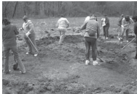
Volunteers excavate a raingarden at Edgebrook Woods, which will grow native plants nourished by stormwater runoff.
